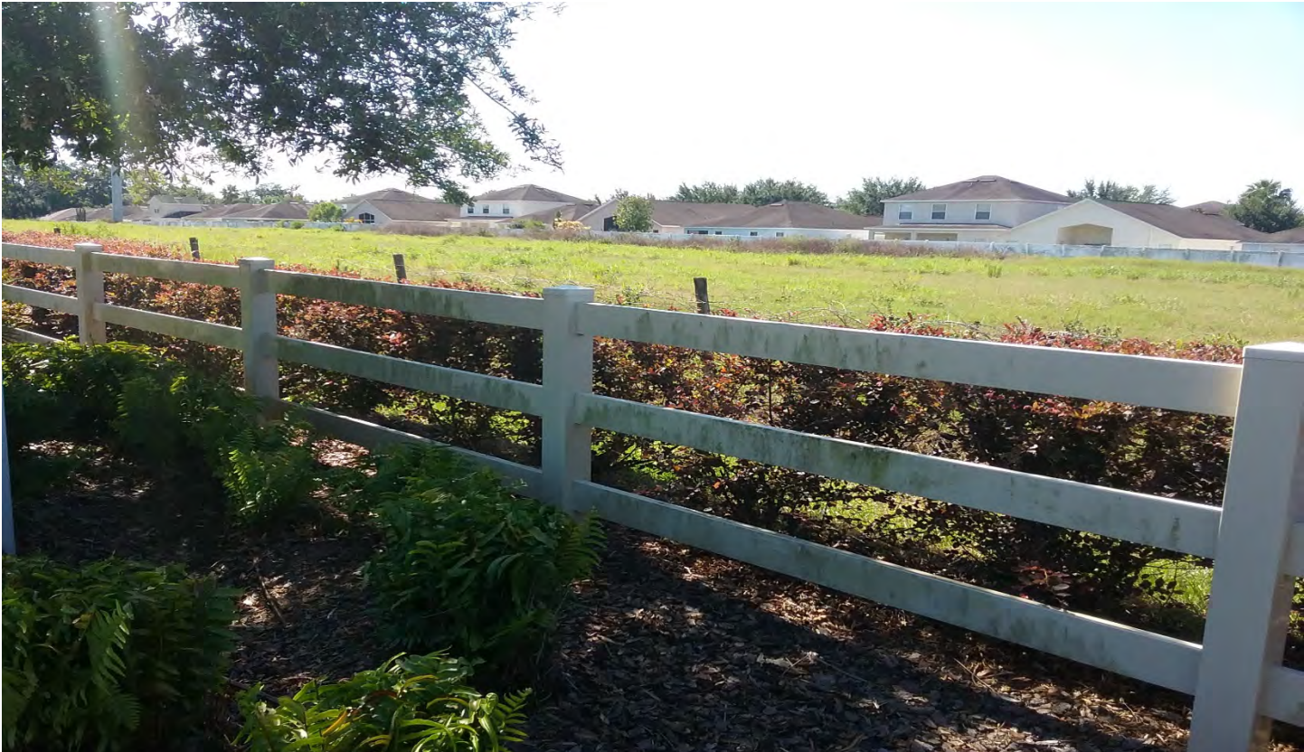
Some areas of the fence along the boulevard needs to be pressure washed.
